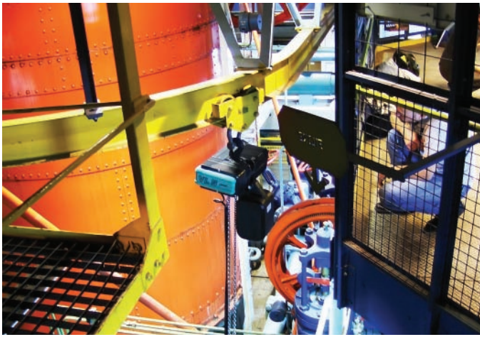
Fig. 6. Another view of the sub-basement equipment with a portion of the large orange accumulator on the left. Credit: France Languérand.
